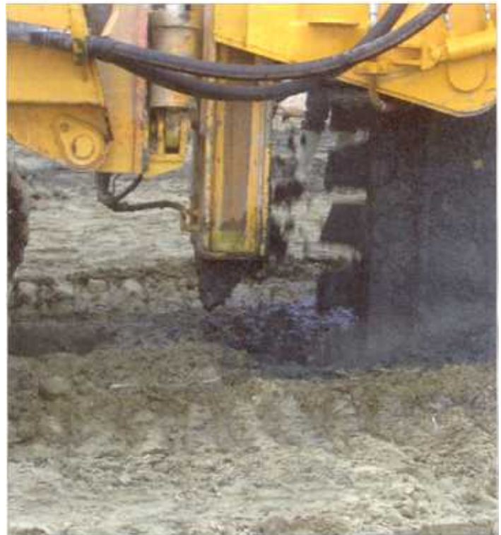
The Trenchmix system uses a drainage trencher specifically modified to break up and mix the soil
